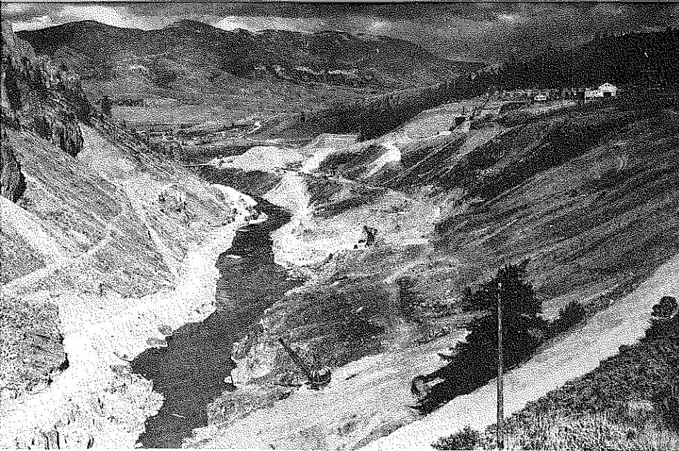
▼ Fig. 3. Green Mountain dam site looking upstream. Talus slopes on left, glacial drift on right. Shows stripping operations in glacial drift and Morrison-shale. Scaffolding on left is on axis of dam and marks top of gate chamber shaft which starts in upper porphyry sill and ends at tunnel level in Morrison shale.
