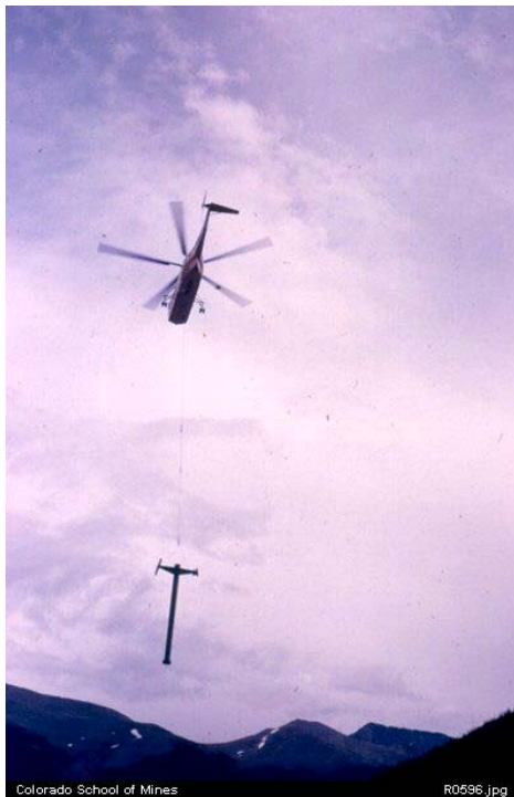
Erecting tower at Copper Mountain, Colorado Photograph by Charles F. Dwyer July 1972
