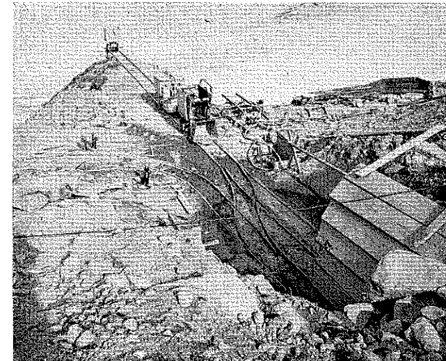
Figure 2. Tunnel surface facilities, showing haulage track, mucking machine, battery locomotive, mine car, and disposal dump.
