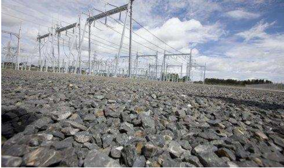
Figure 4.16 Typical Crushed Rock Used to Increase Surface Resistance
