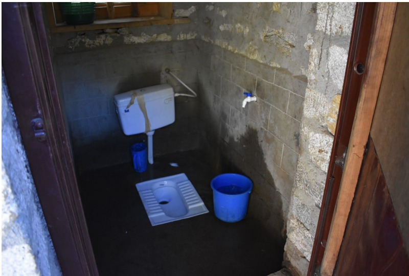
Pour flush latrines are extremely common along the Everest Base Camp trail. These facilities often discharge out the back of the buildings without treatment.
