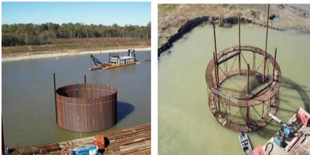
Figure 4.11. Installation of wale and strut system and driving the sheet piles (Nemati, 2005).
