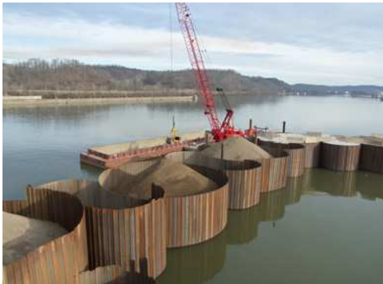
Figure 1.1. In-water construction of a cellular cofferdam (photo from C.J. Mahan Construction Co).
