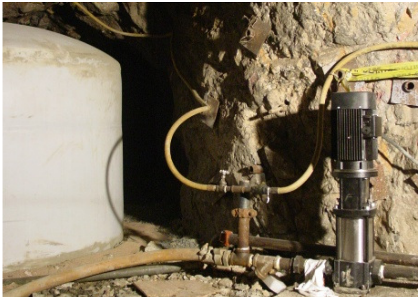
Figure 4.5 Water reservoir and priming pump
