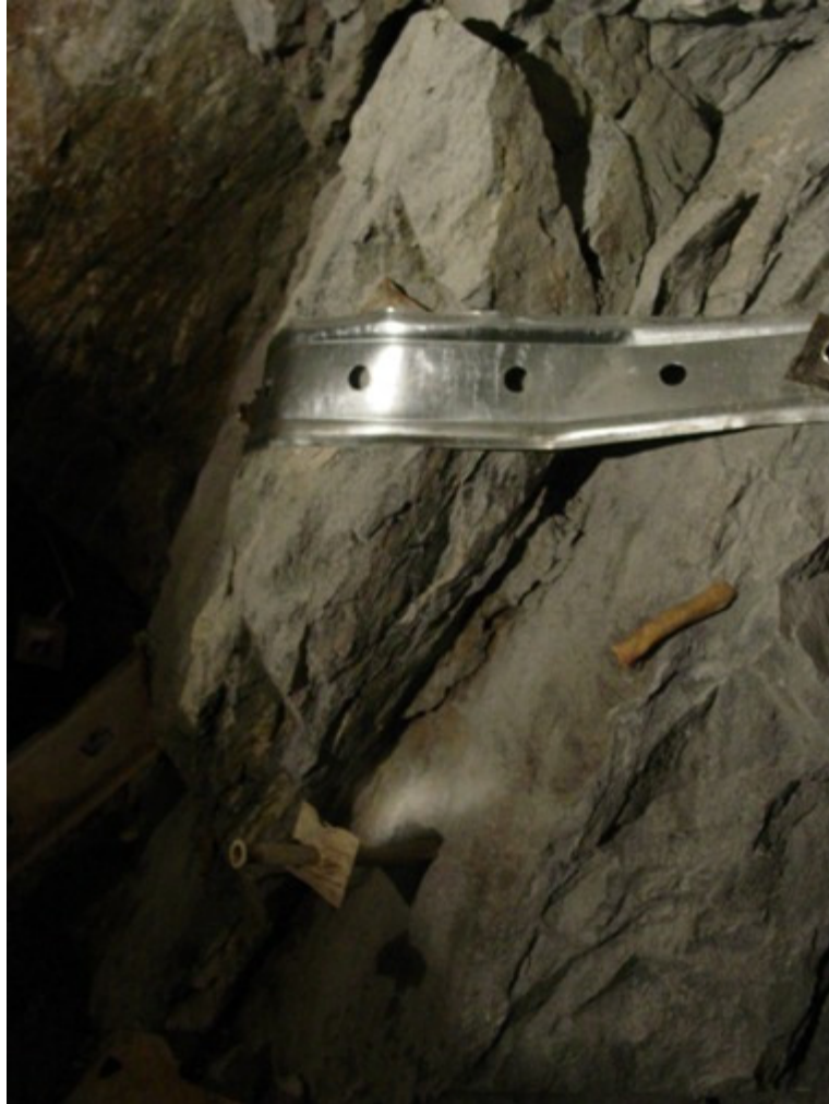
Figure 6.39 Large slab bound by open discontinuities
