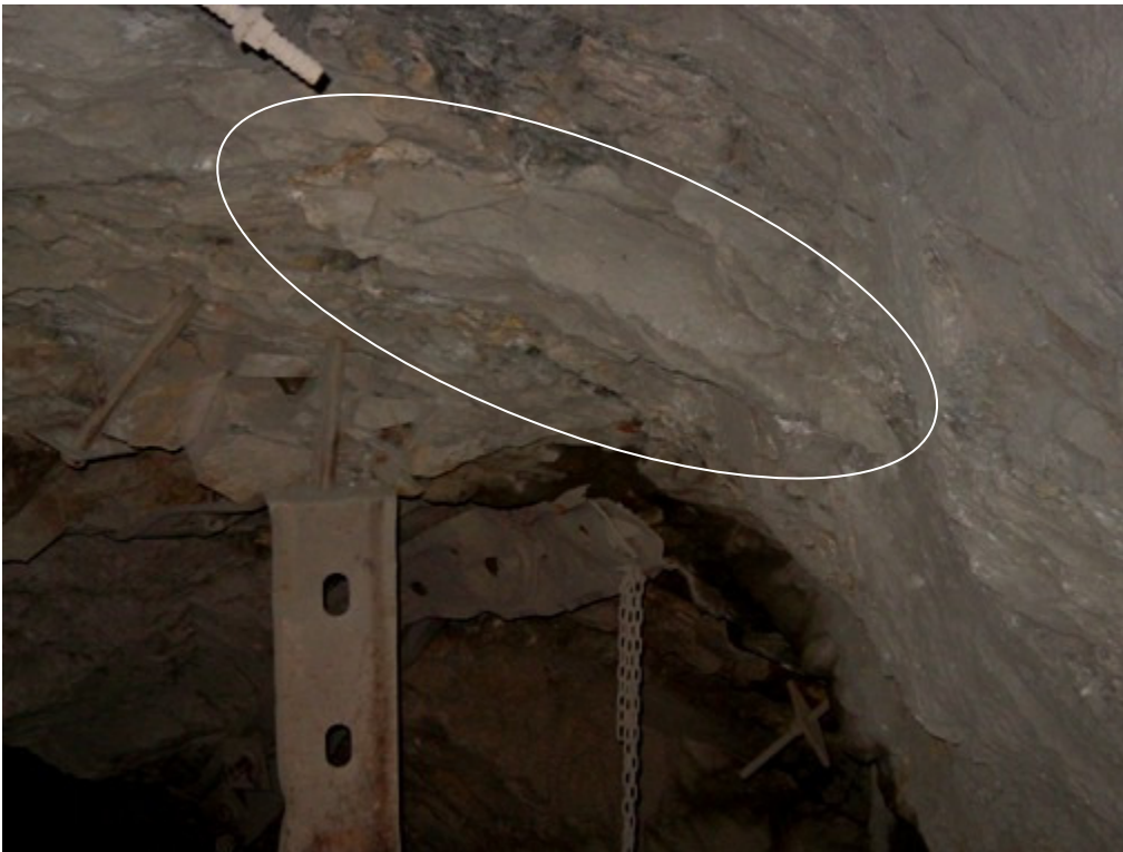
Figure 6.34 Fractured material in north east corner
