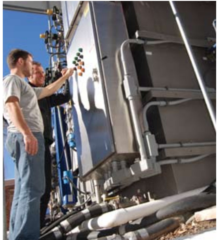
Jörg Drewes and Rick Huggins adjusting the control panel of the bioreactor.
