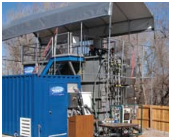
AQWATEC’s bioreactor located in Mines Park.
