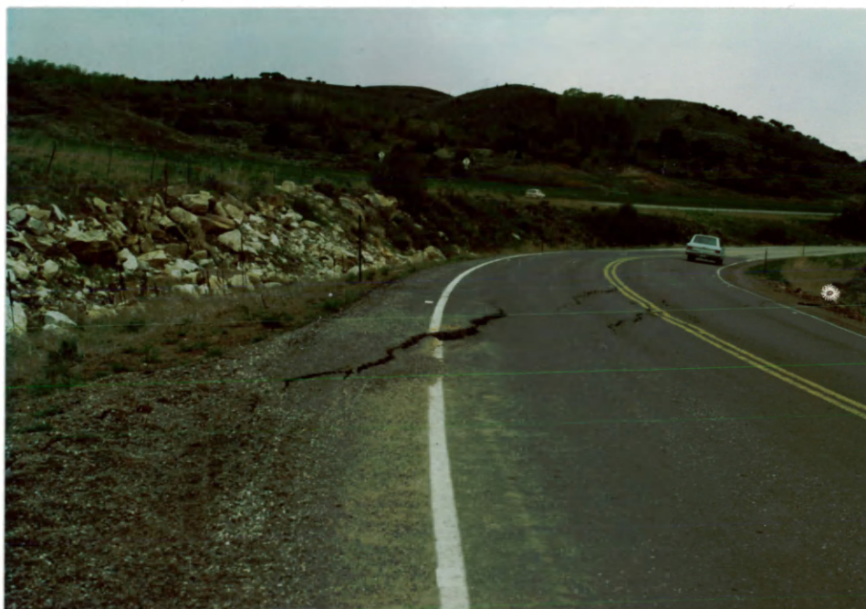
Figure 19 : Combined Vertical and Horizontal Movements on a Crack along Highway U.S.6 at the Western Margin of the Slide.
