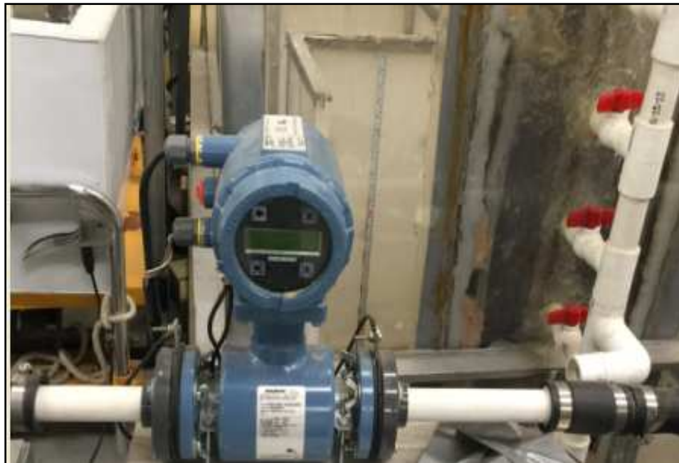
Figure 3.5: Flow meter used to monitor the slurry flow.
