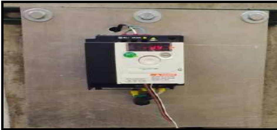
Figure 3.6: Variable Frequency Drive (VFD).
