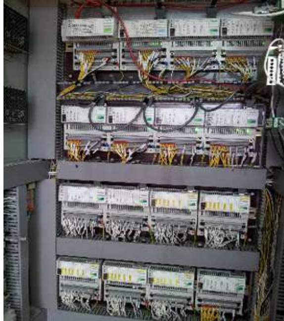
Figure 1.6: The sample image of Programmable Logic Controller (PLC)
