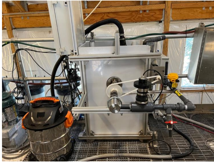
Figure 2.2 Cloth media filter system installed at Mines Park water reclamation station.
