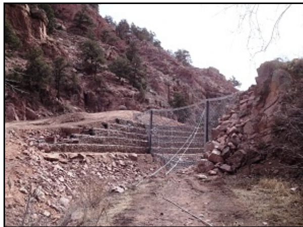
Fig 6. VX net (below) and UX net (above) with armored access abutment, Glen Eyrie Conference Center, Colorado Springs, Colorado.
