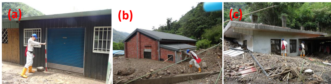
Fig. 3. Damaged building and damage class applying Jakob et al. (2012) method: (a) #4, metal sheet structure with damage class I; (b) #11, brick structure with damage class II; (c) #13, reinforced concrete structure with damage class III (photo: Hsu, C.H.)
