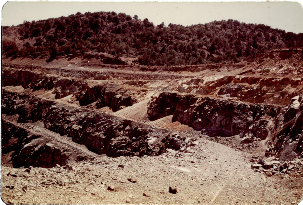
Figure 97. A typical wedge failure involving sliding along the line of intersection of normal fault and joint planes. Location: west wall of the pit.
