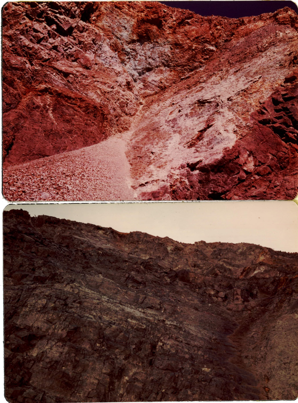
Figure 102. Sets of intersecting normal faults and joint plane gave rise to the formation of wedge failures. Location: two different cases in the west wall of the pit.
