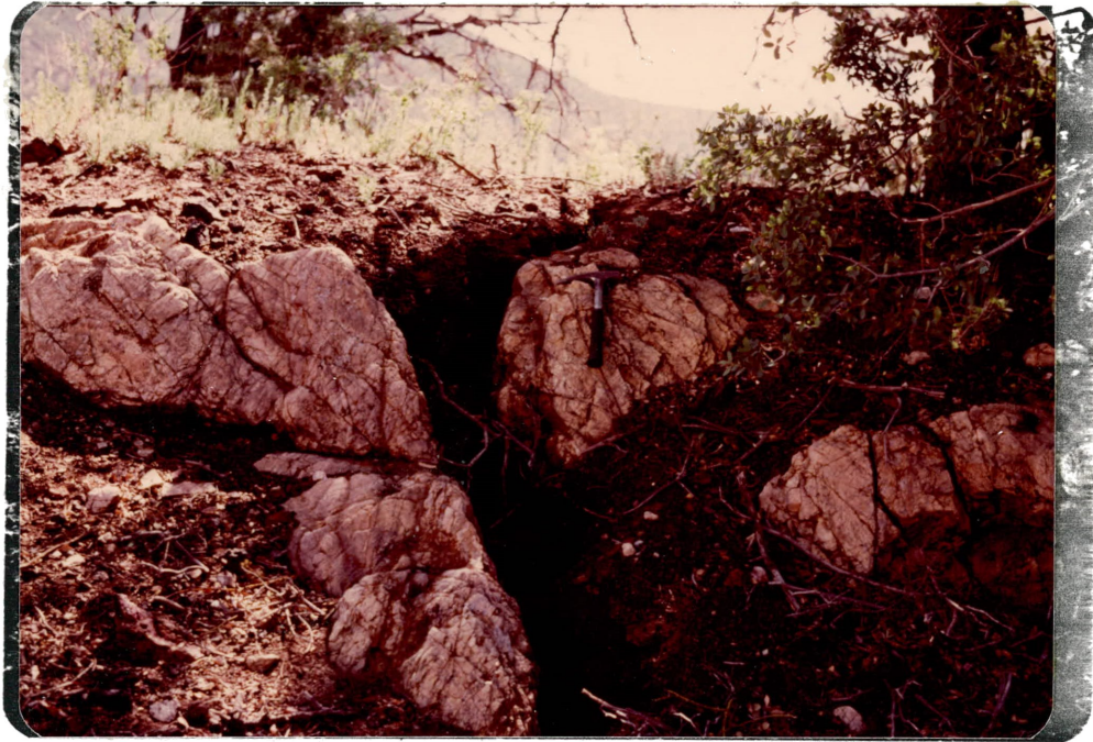
Figure 104. Tension crack showing some part of a top tension crack in the foot-wall of the Barringer fault (south wall). Considerable horizontal and vertical movements have occurred. Looking west.
