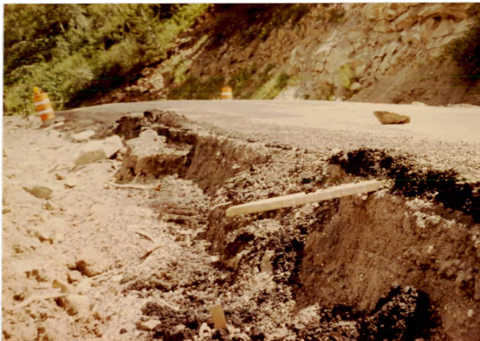
Figure 16. Before and after shots of a measurement point along the south lateral scarp on the highway. The top photo was taken May 14, 1985, and the bottom photo was taken July 31, 1985.
